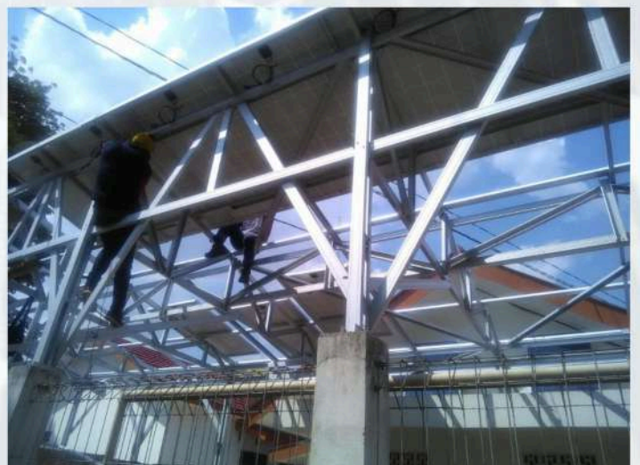
Solar On-Grid System-UNSRI (Palembang)
