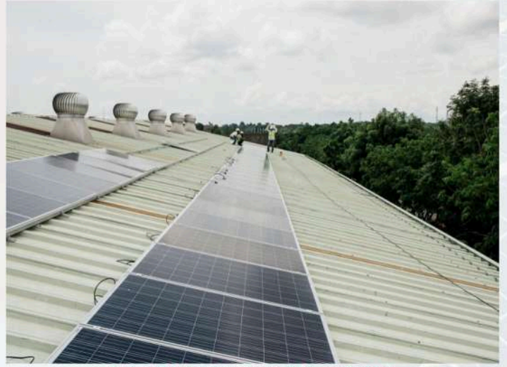
Solar On-Grid System-Philips Batam
