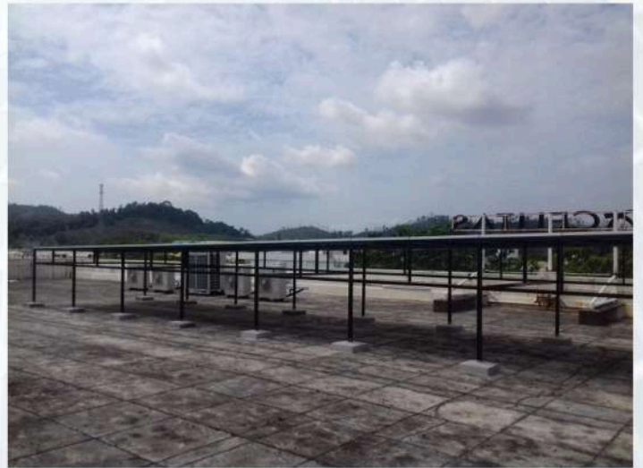
Solar On-Grid System-Excelitas Batam
